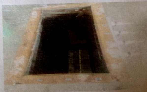
Transformer Insulating Oil in Tank
