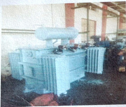
Whole Transformer setup
